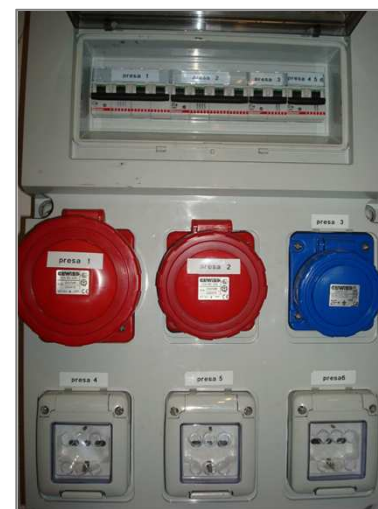
Main circuit breaker box
